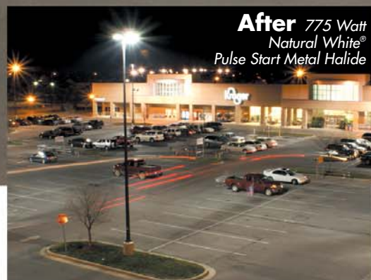
Before 1000 Watt HPS
